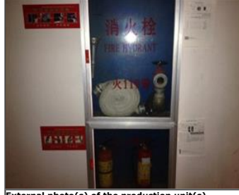
External photo(s) of the production unit(s) Fire extinguishers and fire hydrant in the dormitory.JPG
