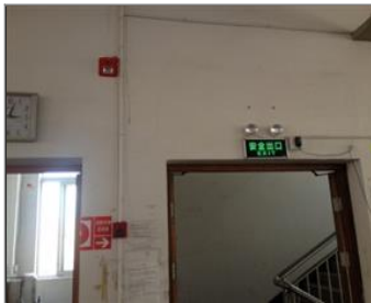
External photo(s) of the production unit(s) Exit sign, fire alarm and emergency light.JPG
