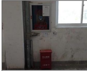
External photo(s) of the production unit(s) Fire extinguishers and fire hydrant.JPG
