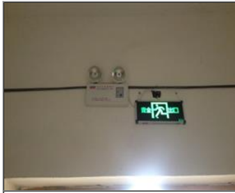
External photo(s) of the production unit(s) Emergency light and exit sign in the dormitory.JPG
